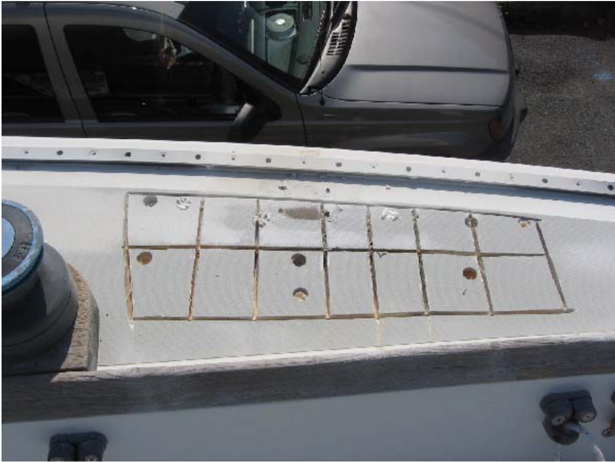
Stanchion removed and a hatch pattern cut to facilitate removal of old core. Cuts using a 4.5 inch angle grinder
